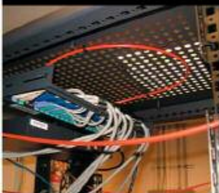
Firetrace does not occupy valuable rack space. This red Firetrace Detection Tubing is run unobtrusively across the top of the rack.
